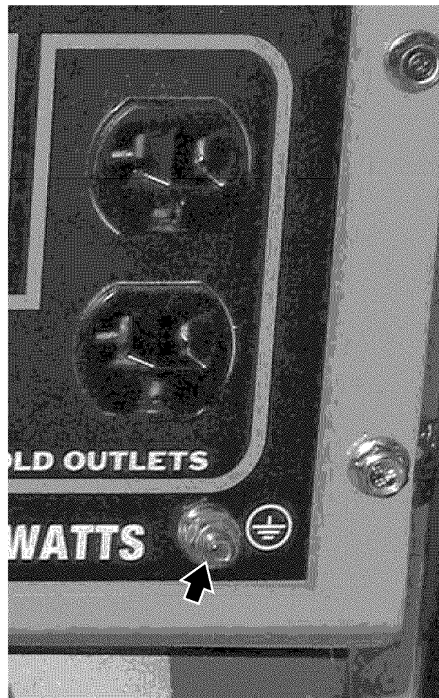
Figure 19 – Ground Terminal on the Control Panel
